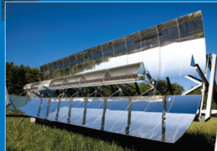
Close-up of a parabolic trough showing collector tube containing oil at trough focal point.
