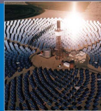
This 10-MW power tower facility known as Solar Two near Barstow, California, demonstrated molten salt storage.
