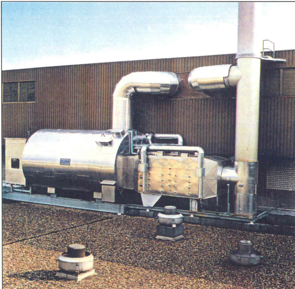
Compact unit with thermal oil boiler
